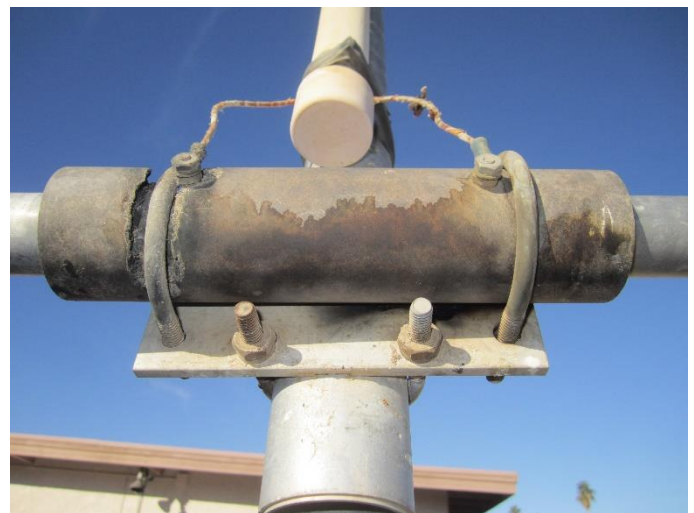
Why is this a lucky break for K6LL? A short from boom to U-bolt through the burned insulator turned out to be intermittent and Dave was able to finish the contest before discovering the extent of the problem. (Photo credit, Dave Hachadorian, K6LL)
