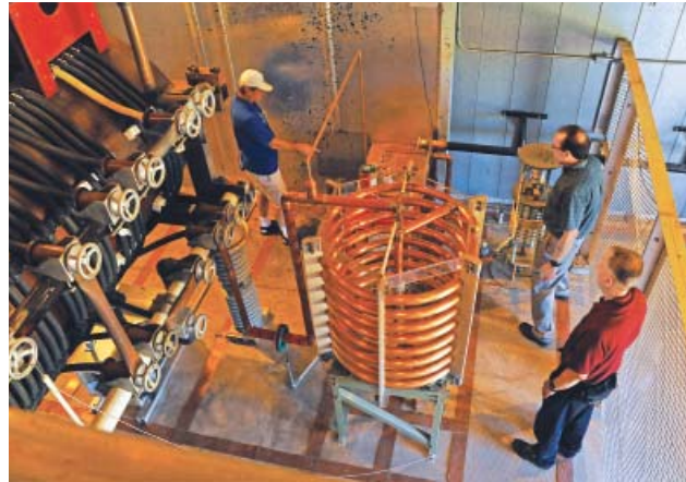
The helix house that powers WWV's antenna array.
