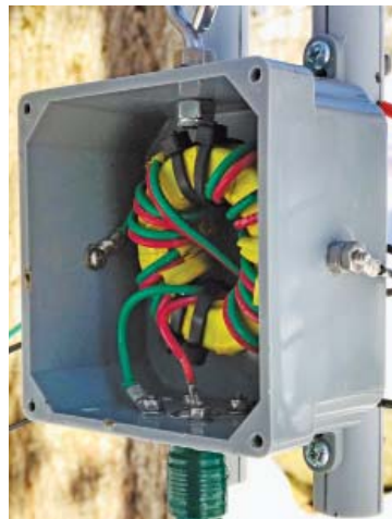
Figure 3 — The feed-point box with the balun installed and PVC spacers attached to the box-mounting tabs.
