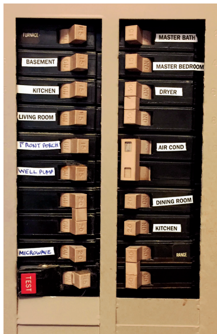
A typical circuit breaker panel with labeling. With your portable radio at hand, start turning off the individual circuits until the interfering signal disappears. If turning off the “Living Room” breaker, for example, kills the signal, your culprit is hiding somewhere in that room.
